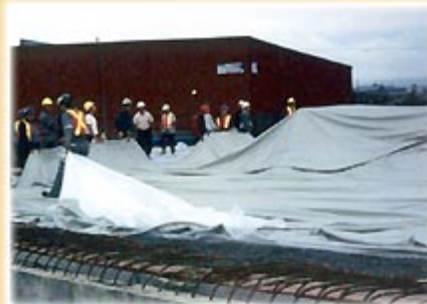
2. The airform is attached to the exterior of the ringbeam. The airform is prefabricated to the dimensions of the building and delivered on site ready to inflate.
